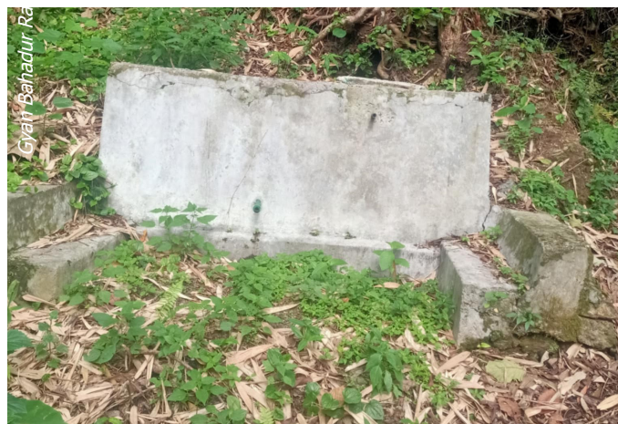
A water tap is in ruins due to neglect and lack of ownership
